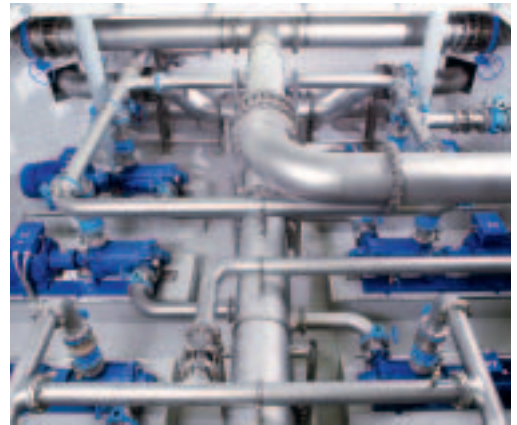
Distributed pumping stations are networked to each other and data is thus exchanged via easyNet.
