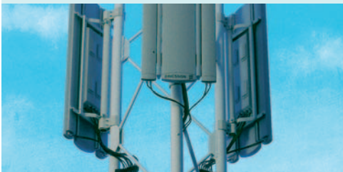
in transmitter stations of cellular phone networks
